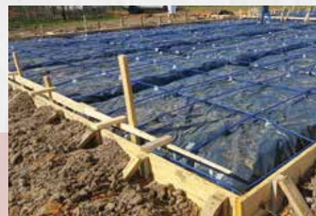
PE Unbonded Post Tension (Flooring)
